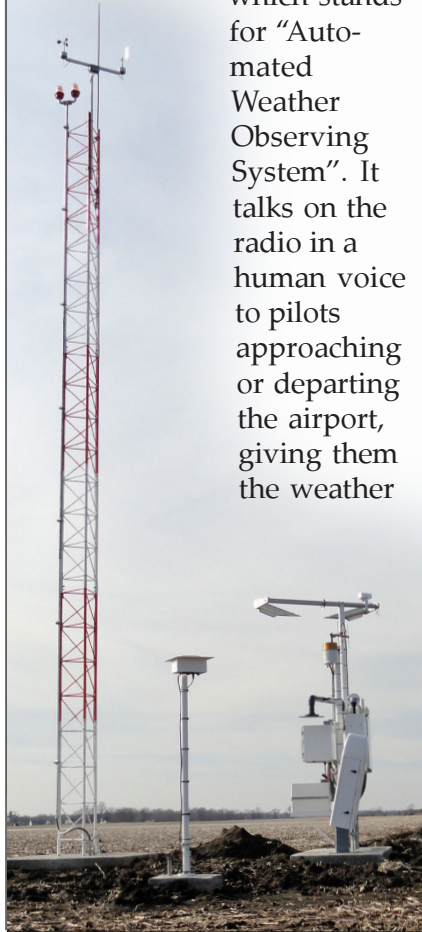
On-airport AWOS station measures weather and broadcasts to pilots.
